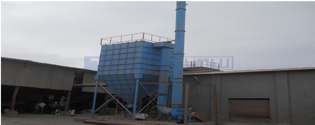
Figure.4. Dust suction and filtration unit (Tech flow, 2002).
