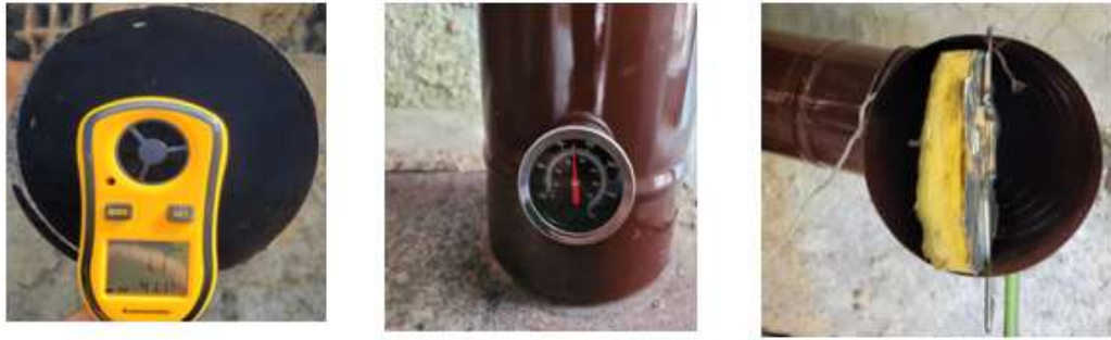
Air velocity measurement at the main chimney outlet
